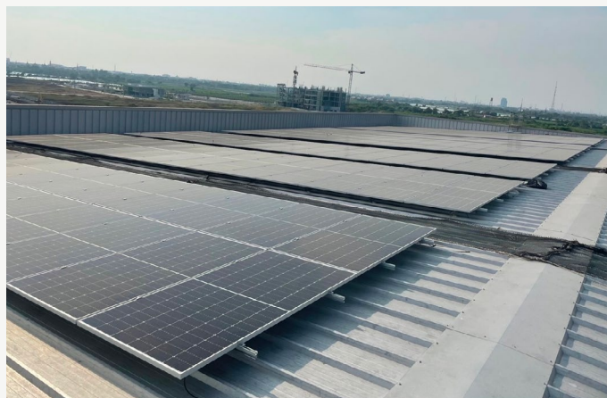
Solar panels installed on our factory
