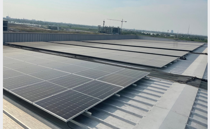
Solar panels installed on our factory
